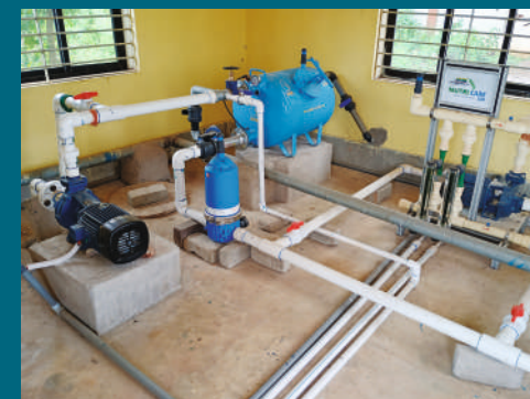
Water filter unit
