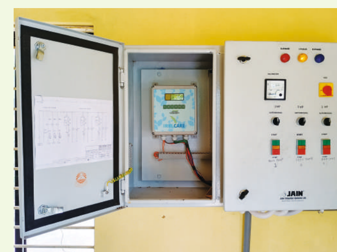
Sensor panel for drip fertigation
