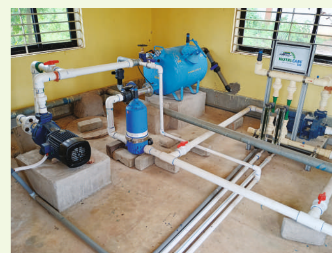
Water filter unit
